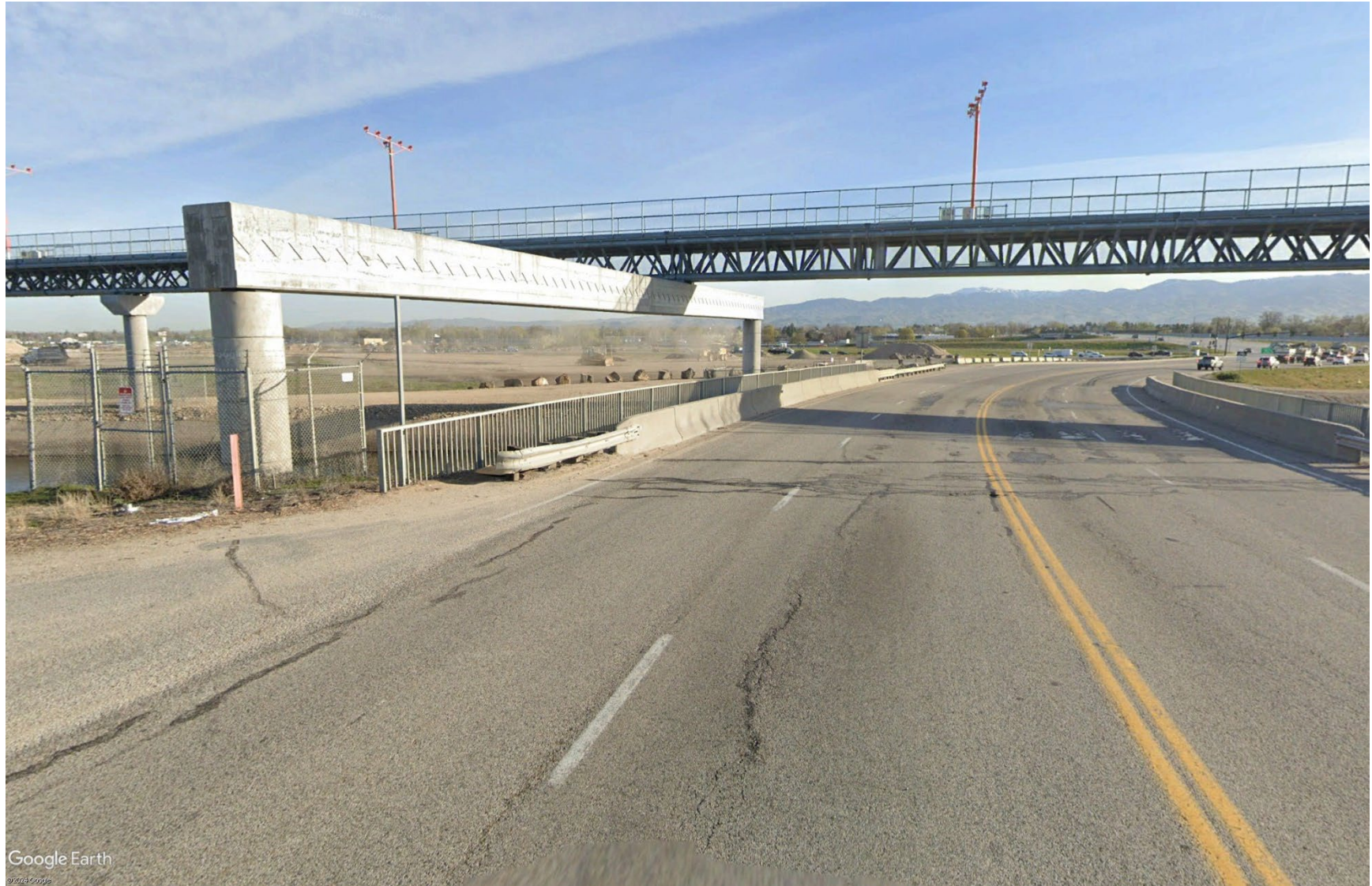
Figure 2 Picture of Bridge over New York Canal showing ALSF-2 Lights, Concrete Girder, and Support Column
